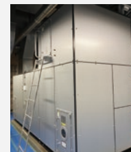
Air handling unit
